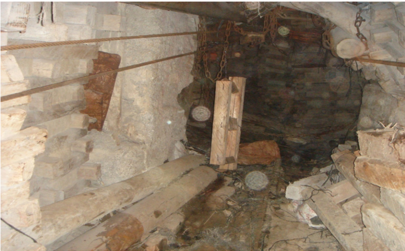
Figure A18: A Timber Pack Being Conveyed to the Stope by the Mono-Winch
