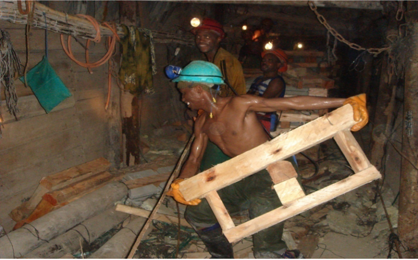
Figure A15: Team Workers Clearing the Route Via Which the Mono-Winch Conveys Material to the Stope
