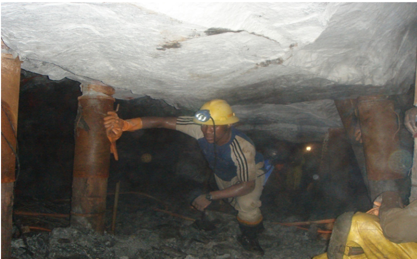
Figure A10: A Stope Worker Inside the Stope. Also Visible Is the Installation of Temporary Support Using Props. Permanent Support Is Installed Using Timber Packs
